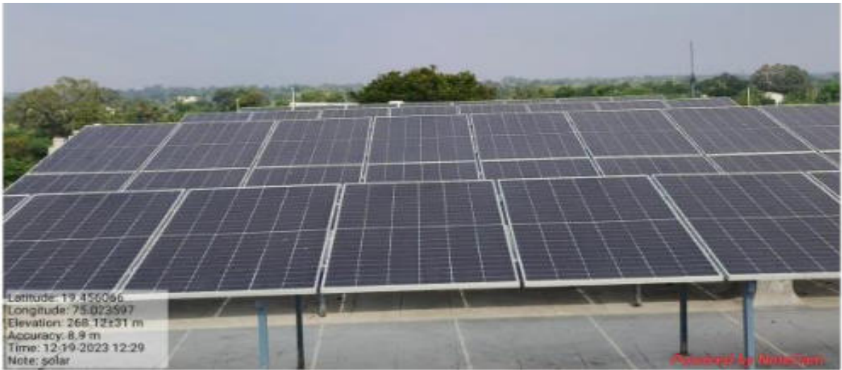
80 kVA capacity solar system
